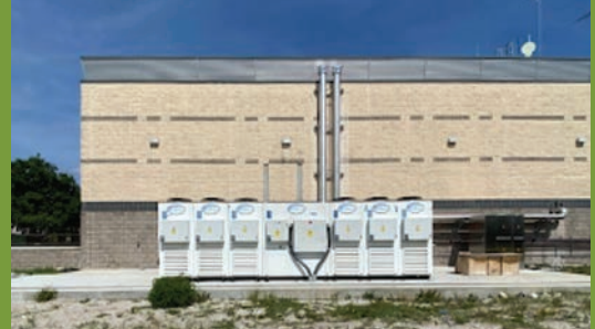
Central HVAC System
