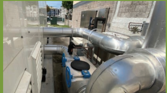
Central HVAC System
